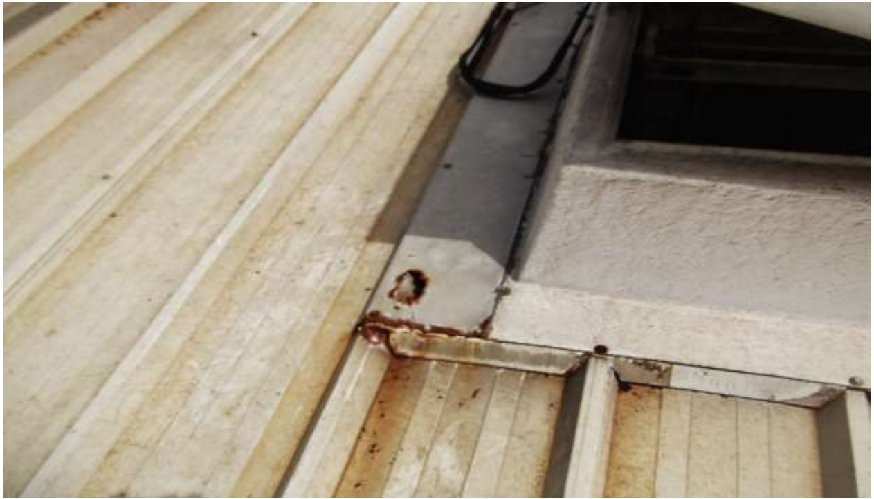
Fig. 9. Rust at connections between rooflights construction and sandwich panels after 4 years on the Production Hall roof.
