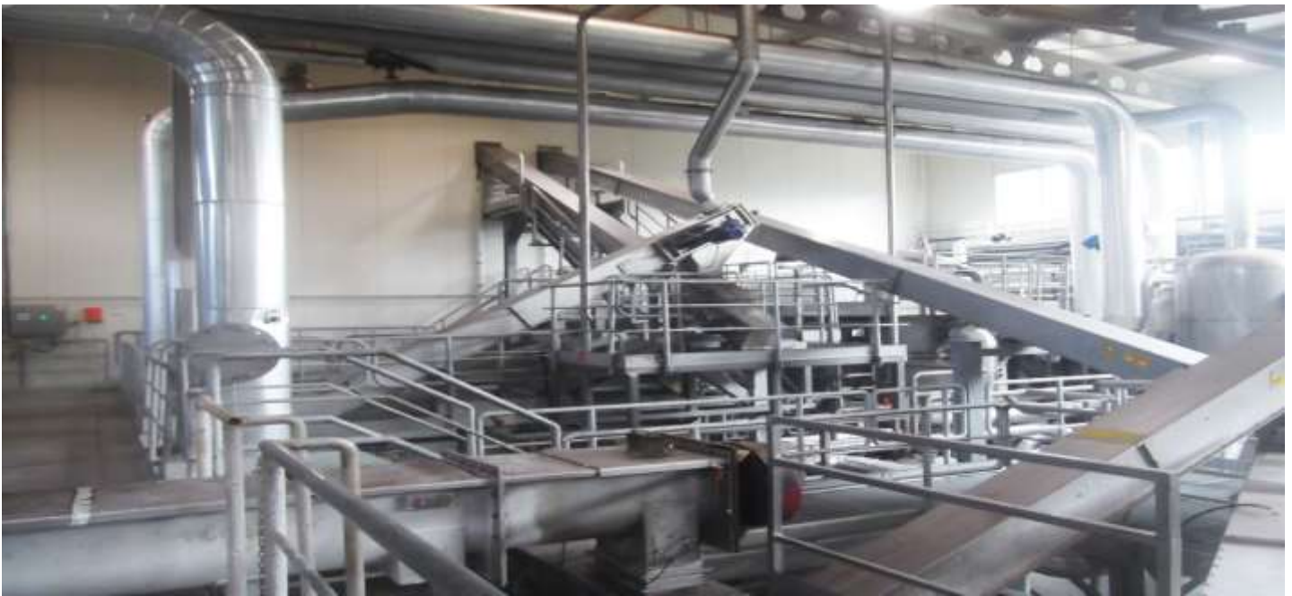
Fig. 1. Galvanized steel constructions in the Production Hall contaminated with poultry meal were free from rust. Aluminium mantels over piping was with no corrosion signs.
