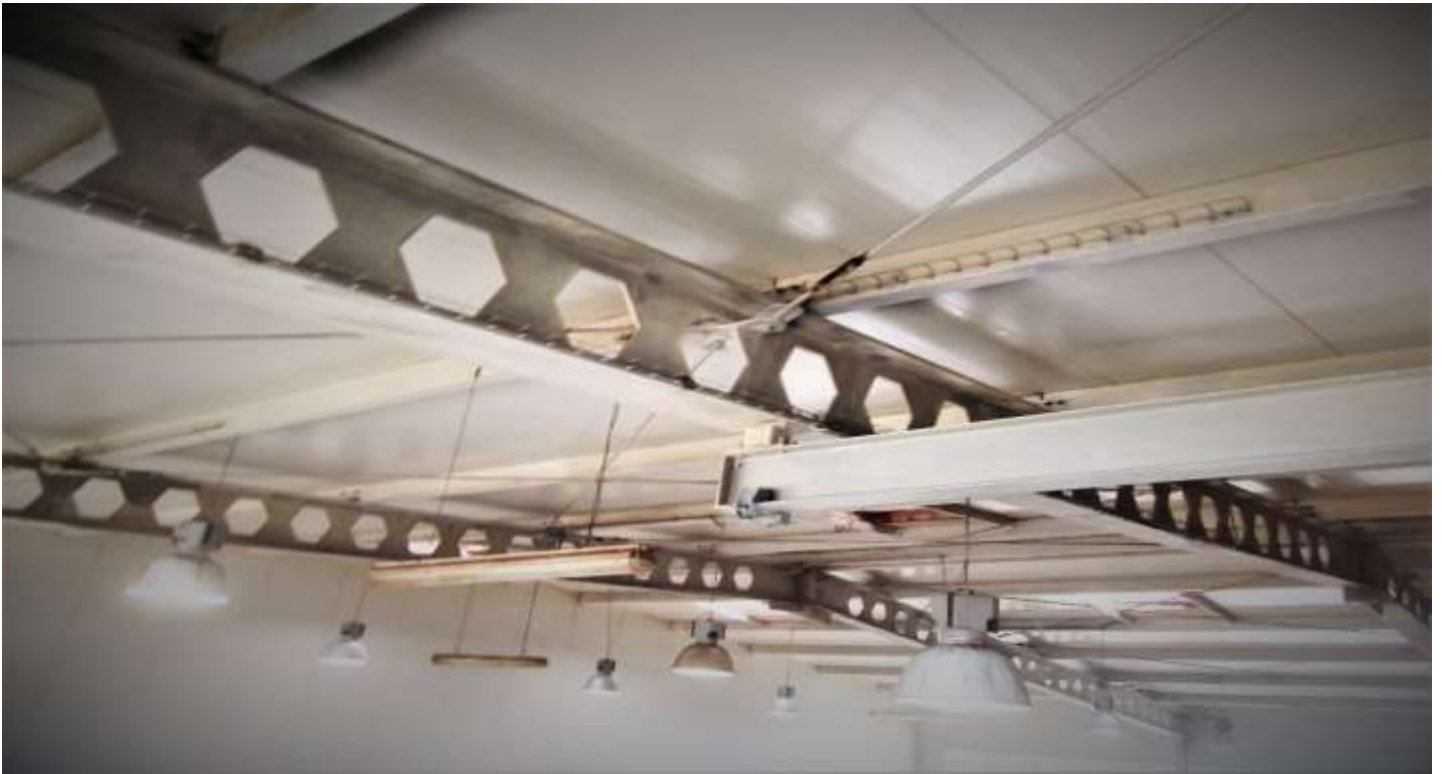
Fig. 6. Threat of corrosion cracking of rusted steel rod threaded parts due to continuous stress.
