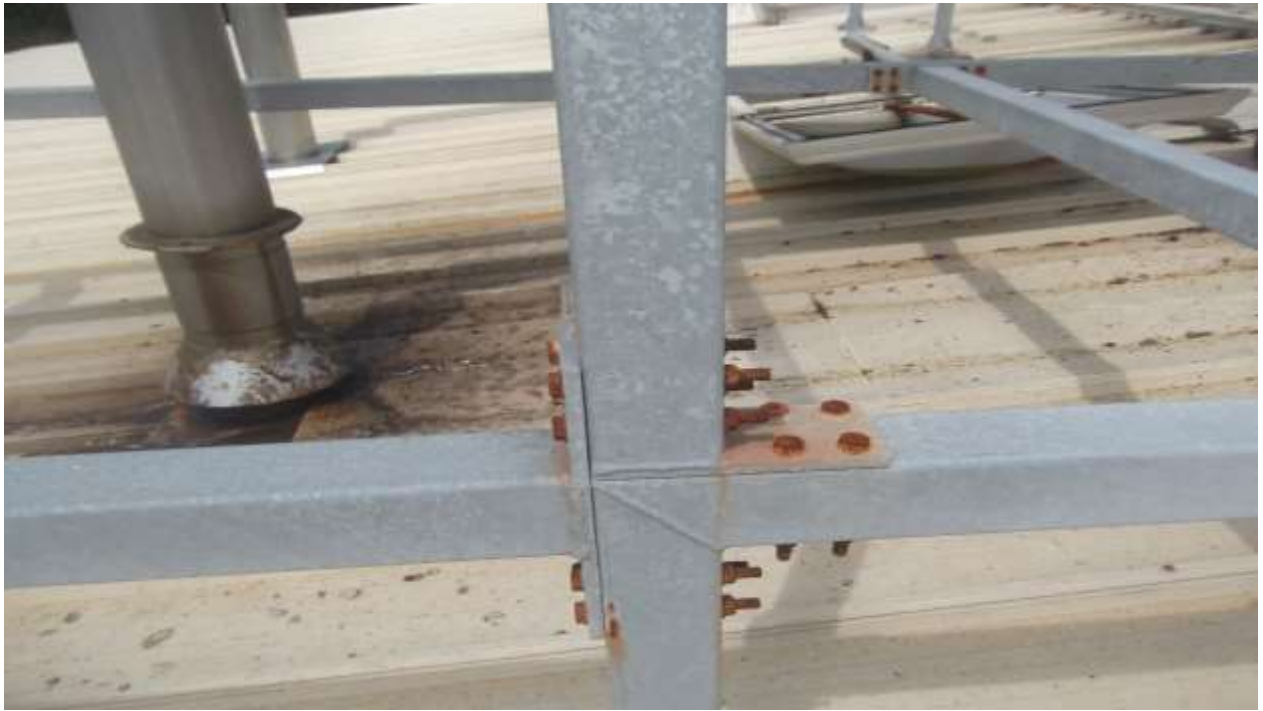
Fig. 11. Galvanized steel structures with no corrosion; steel screws covered completely with rust after 4 years on the Production Hall roof.
