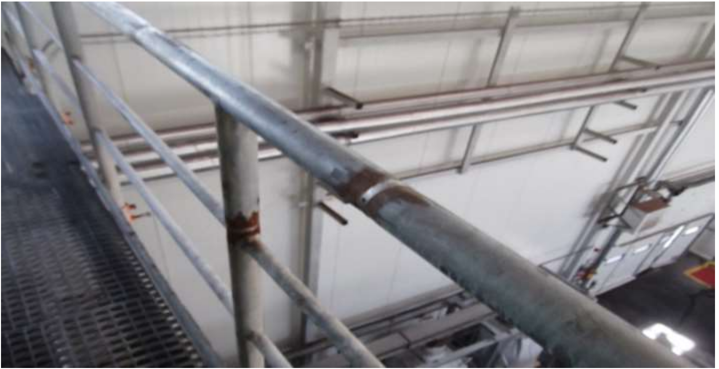
Fig. 4. There were few places on the constructions, for instance after re-welding, covered with rust. Renovation after mechanical cleaning should be done with a paint loaded with zinc dust..
