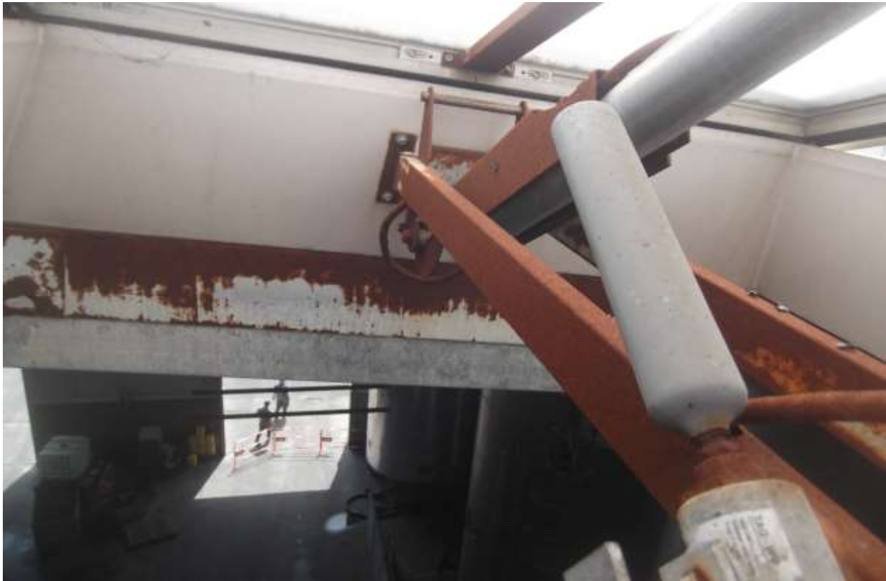
Fig. 8. Elements of dome rooflights with pneumatic locking, used for ventilation, were intensively corroded after 4 years at the Production Hall roof.
