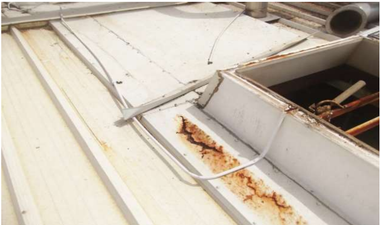
Fig. 10. Painted steel plates and rooflights were locally completely destroyed after 4 years on the Production Hall roof.
