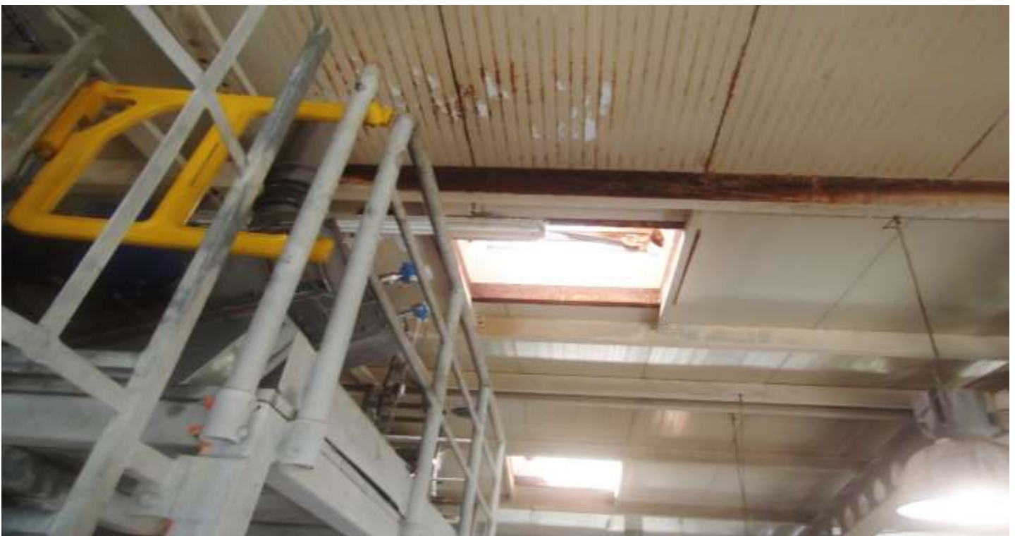
Fig. 5. Corrosion of construction elements including sandwich panels consisting of hard mineral wool core covered with galvanized and painted steel plates rusted within the flow stream of aggressive gases.
