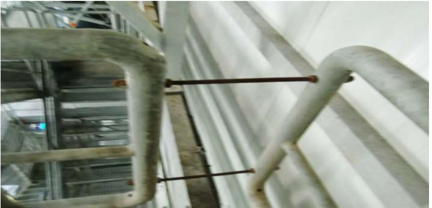
Fig. 7. Rusted rods without protective coatings may be affected by stress corrosion cracking.
